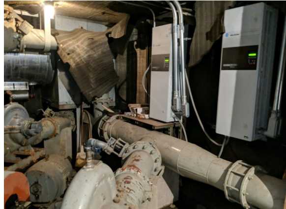
Figure 6-3: Cornell & Pennsylvania Booster Pump Station
