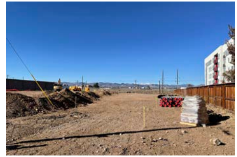
15 A new multifamily housing development is under construction next to Oxford Station Apartments.
