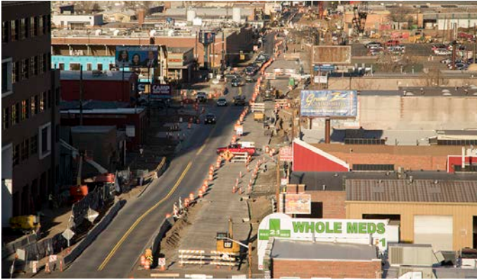
Brighton Boulevard under construction with existing industrial uses next to high rise development. Photo by Kevin Beaty, Denverite.
